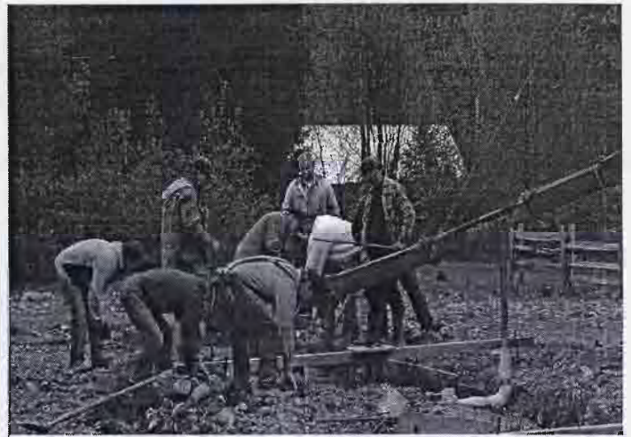
Volunteers at work pouring concrete for footers on new Coffee Creek Fire Hall
