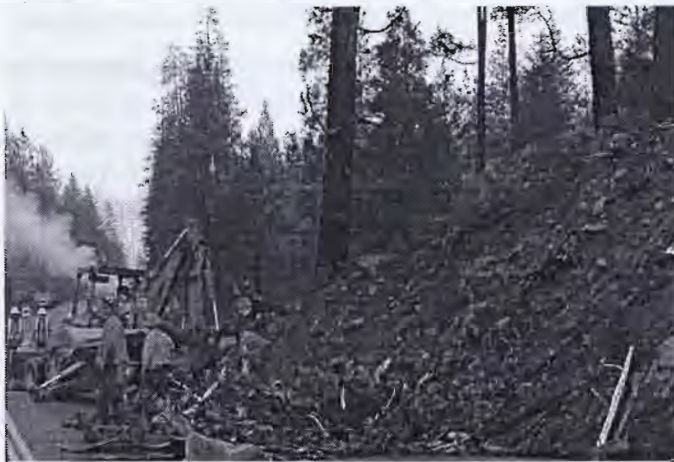
Cal Trans Workers Clean Up Downed Trees
